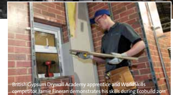
Students learning about drywalling at British Gypsum's Drywall Academy in East Leake
