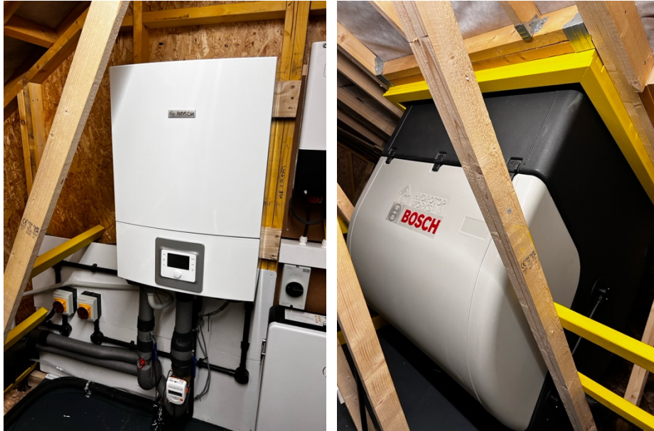
Figure 171. Indoor and outdoor unit located in roof space
