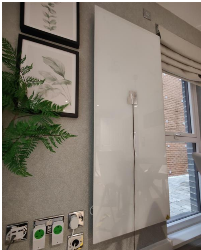
Figure 11. Curv infrared panel
