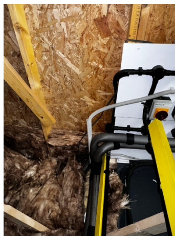
Figure 175. Waste pipe to dispose condensate located in the roof space
