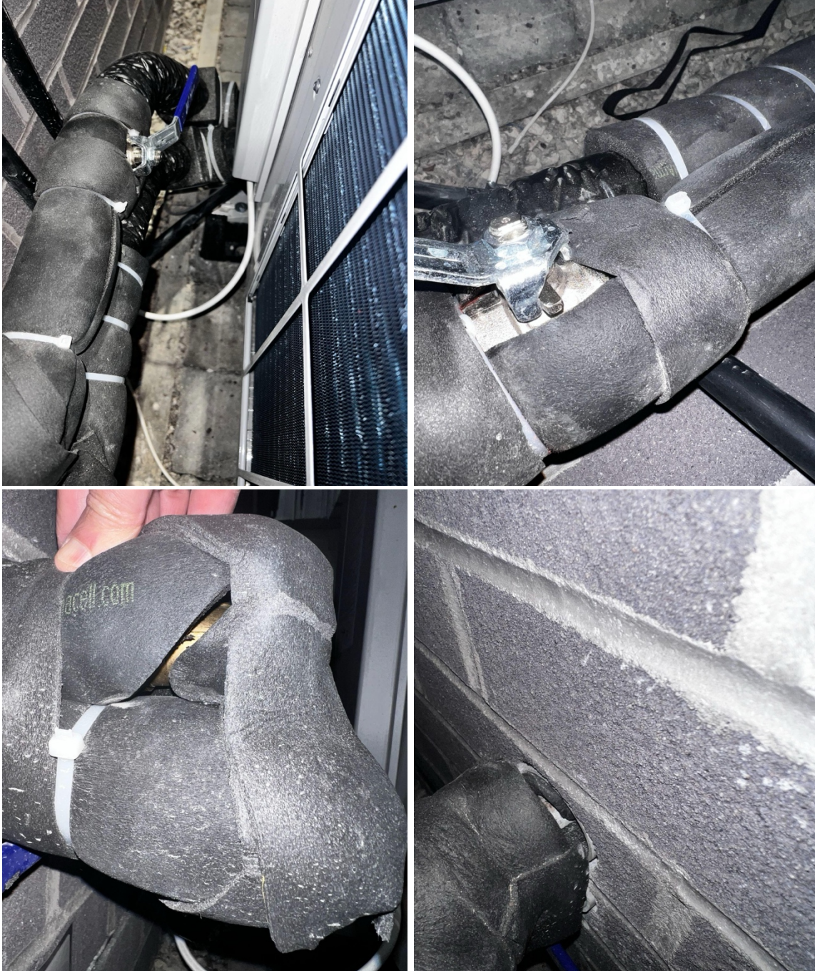
Figure 167. Poor insulation practice externally to the ASHP flow & return pipes
