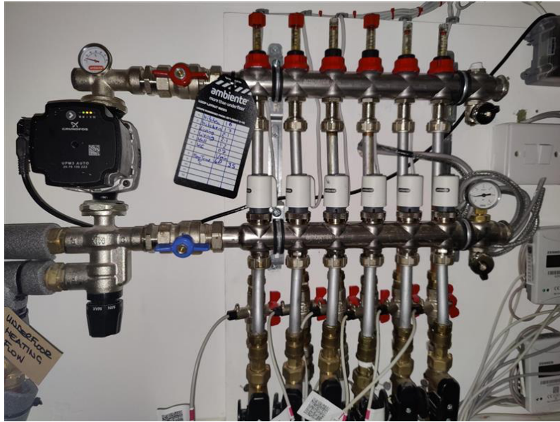
Figure 4. Underfloor heating manifold
