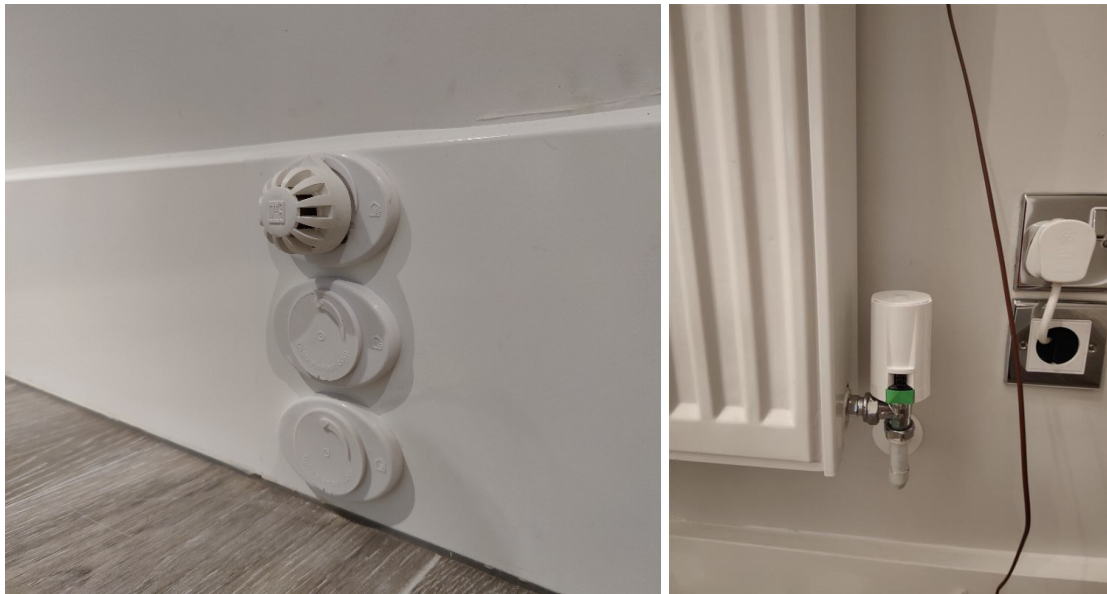
Figure 12. ThermaSkirt control (left) and radiator TRV (right)
