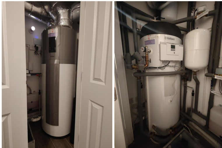
Figure 13. Curv hot water cylinder (left) and Vaillant ASHP cylinder (right)
