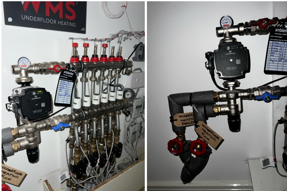
Figure 174. Additional circulation pump
