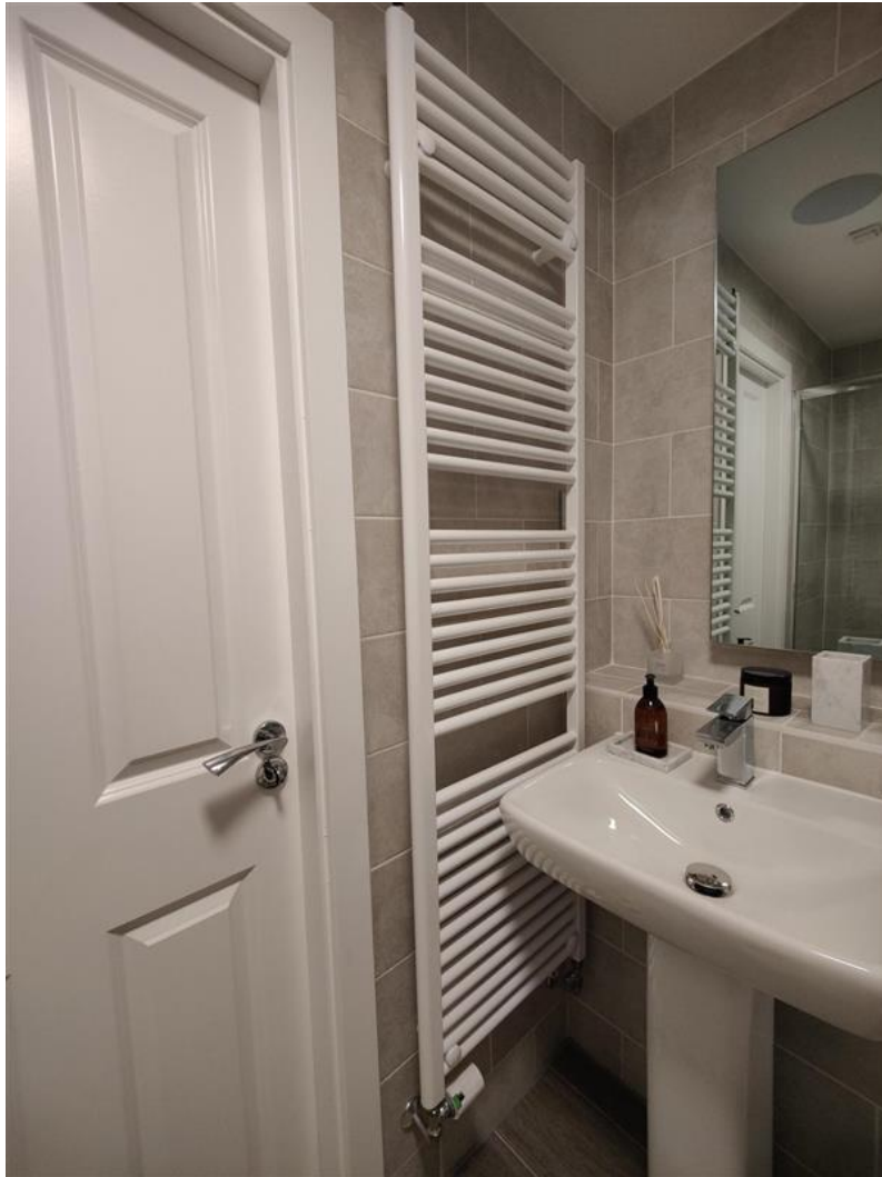
Figure 10. Bathroom towel radiator
