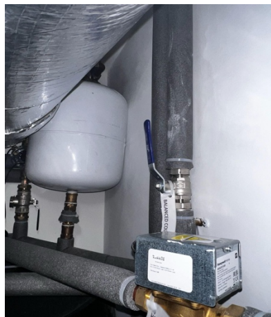
Figure 170. Uninsulated volumizer/solar safety vessel
